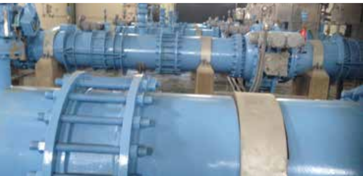
Piping for water plant pumps
